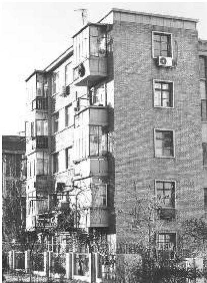
Figure 7 Multi-storey building from the 1970s, Beijing. Poor insulation and air tightness.
