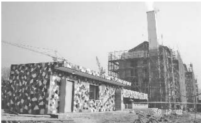
Figure 26 Gas-powered central heating station in Xin Kang, Beijing.
