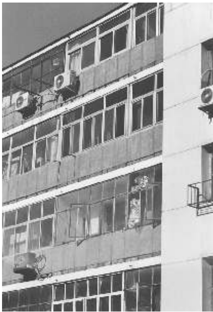
Figure 13 Apartment building from the 1980s. Single-glazed unsealed windows with steel frames.
