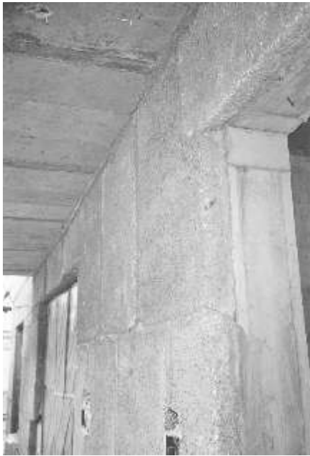
Figure 24 External wall insulation of cement-bound polystyrene blocks, used in part of Xin Kang, Beijing.
