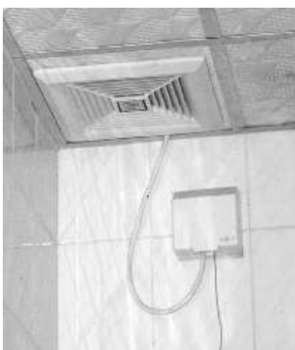
Figure 23 Air exhaust fan in the bathroom.
