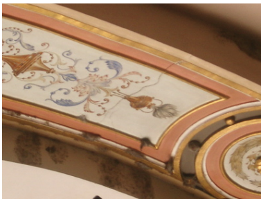
Fig. 10 Fissure on arch
