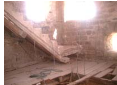
Fig. 11 Unsafe stairs and landings
