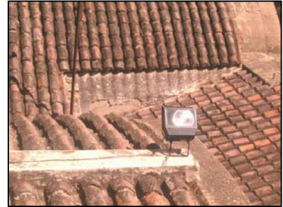
Fig. 7 Detachment of roof material
