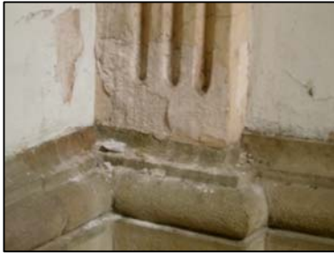
Fig. 9 Dampness and detachment of wall plaster.
