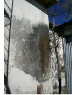
Moisture on the east facade
