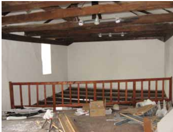
Fig.16 The upper floor of the Stable after the completion of conservation works
