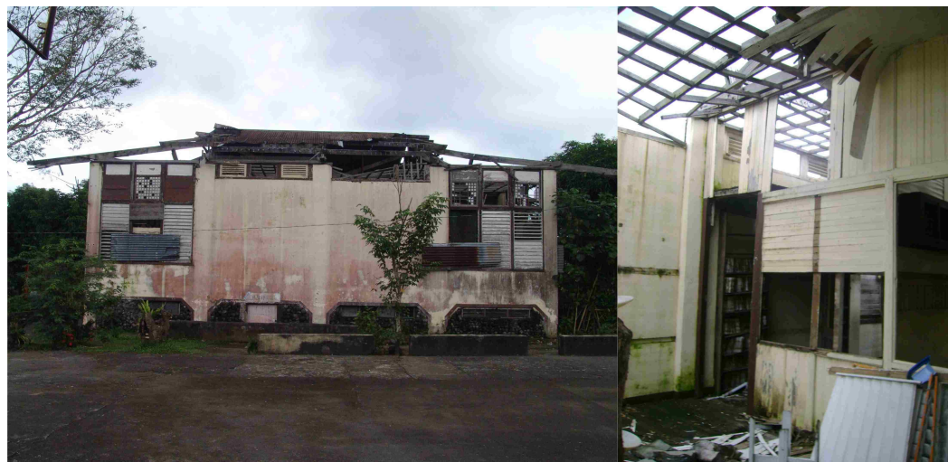
Fig. 7 (left) Back portion heavily damaged while interior (right) is exposed to weather.
