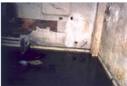
Fig 21, Basement with stagnant water
