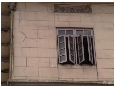
Fig. 35 Cracking of Plaster
