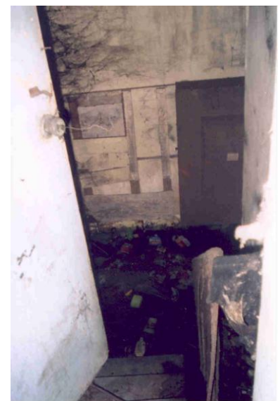
Fig. 37 Basement flooded with water
