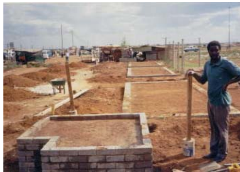
Figure 4 : The construction of the container and watertank bases by a local contractor.
