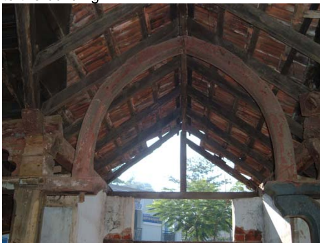
Special timber arches It is a difficult task to find suitable timber for restoration
