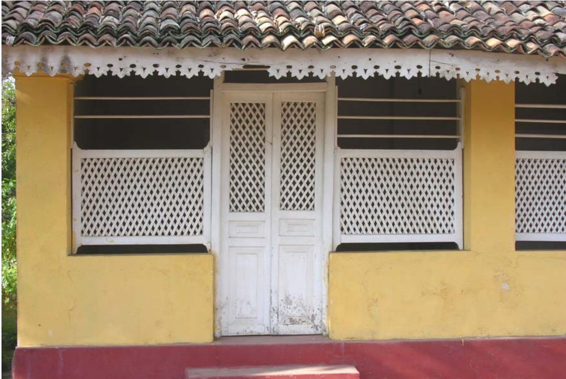
Decorative valance boards, trellis work and the half-round tiled roof emphasize the colonial character
