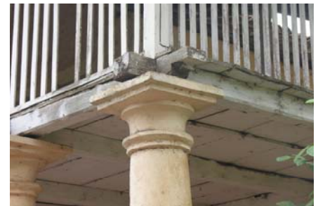
Fig. 43. A timber balcony with loose floor boards and missing elements.
