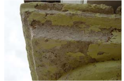
Fig. 42. Dutch lime plaster is peeling off due to salt.
