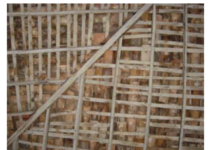
Fig. 44. Present conditions of most roofs.
