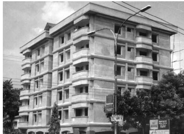
A view of one of the newly constructed apartment building. Only the structural part is completed
