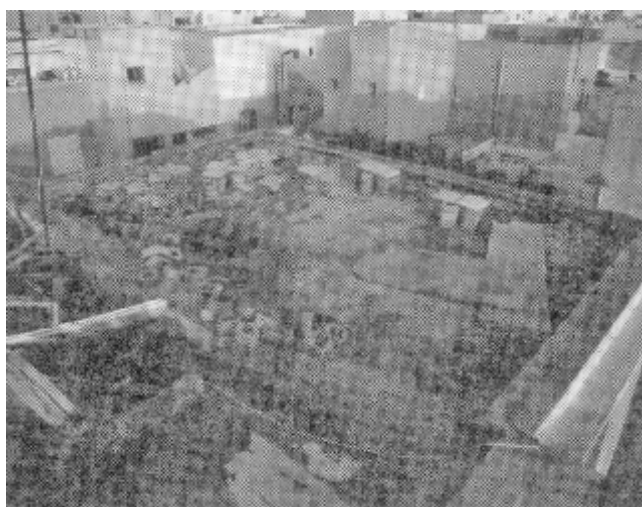
Flat roof covered with scrap which hinders rain runoff and leads to water leakage.
