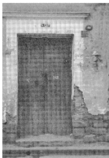
Render falling off the wall and moisture damaged door show lack of maintenance.
