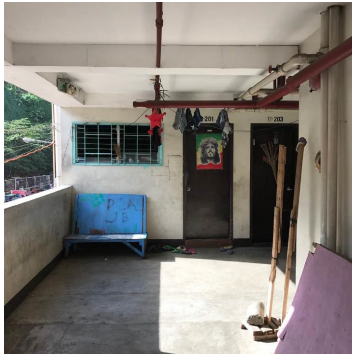
Exterior wall as part of the ‘absorbed screen’, Taken by author, February 2017
