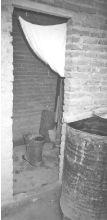
Toilets with no connection to a sewer system.
