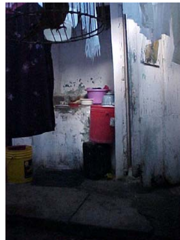
Humidity problems due to leaking roof structures.
