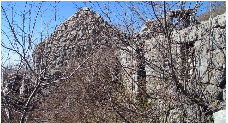
Figure 13 | Deterioration of the site
