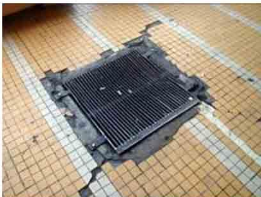
Photo 78. An area drains catch basin. Tiles abounding drain should be replaced and repaired.
