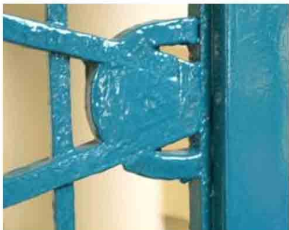
Photo 60. Quality of paint job used for the steel grille of the left wing rear entry. Should be painted discreetly.
