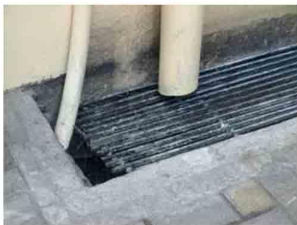
Photo 61. Close-up of external downspout to area drain catch basin. Should be cleaned.
