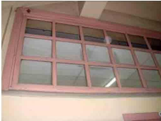
Photo 20. Original fixed wooden casement glass high window is retained at the GF Computer Lab Room. Similar type was removed because of "anay" infestation.
