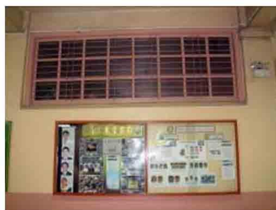
Photo 20. Original fixed wooden casement glass high window with steel grille works. This should be preserved.
