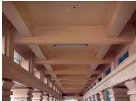
Photo 75. The original Art Deco ceiling with fluorescent lamp used for lighting. Art Deco style luminaires should be added for a more aesthetic appeal.
