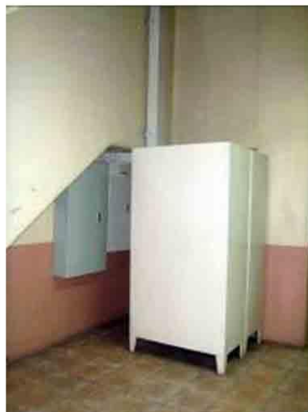
Photo 25. Utilitarian equipments placed indiscreetly near stairway. Should be covered from view.
