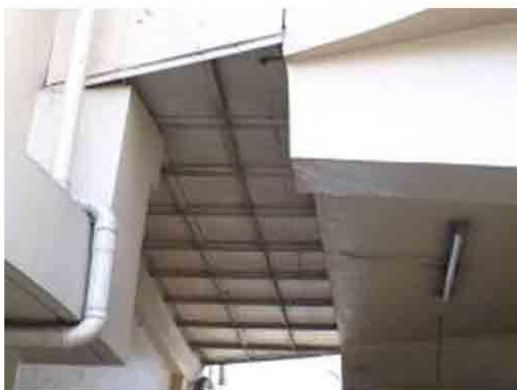
Photo 4. A closer view shows steel frame connector between NRH and Science Building. Should be treated with aesthetic element.
