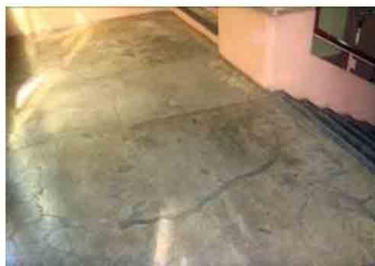
Photo 40. Original cement plaster finish of stairway landing shows remedied patches of cracks.
