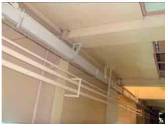
Photo 22. Electrical raceways and air conditioning ducts align the GF ceilings of NRH.
