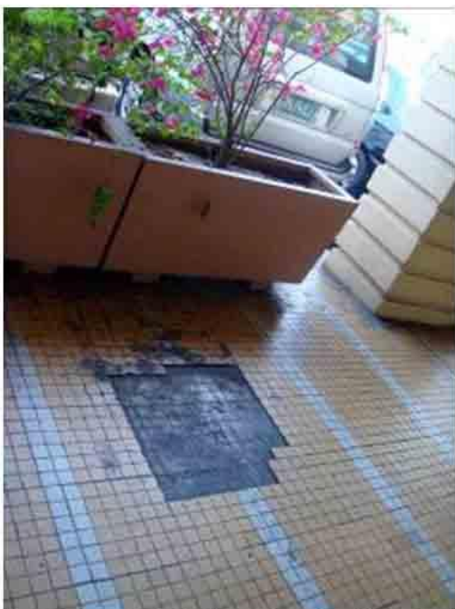
Photo 79. A neglected part of the arcade flooring with original tiles missing. Note also of wooden plant boxes lined along the arcade sidewalk. Should be replaced.
