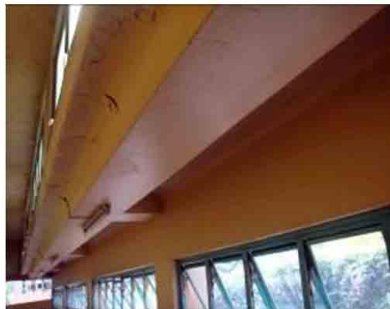
Photo 38. Paint cracks and peels at the bridge way ceiling
