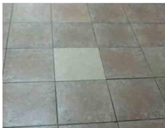
Photo 19. Incompatible color of tile used as replacement
