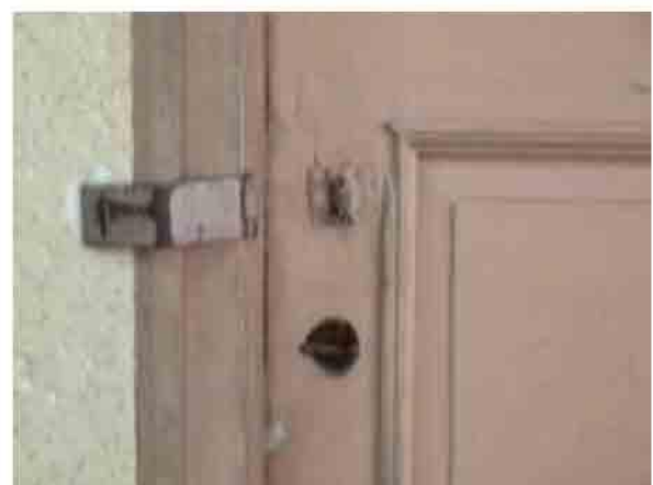
Photo 46. Present condition of an original wooden panel door of one of the classrooms. Should be restored.
