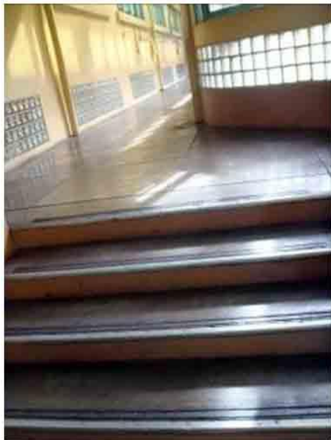
Photo 35. The concrete steps leading to the bridge way show original plain cement finished floor. Original steel bar and aluminum used on stair nosing for skid protection. Should be preserved.
