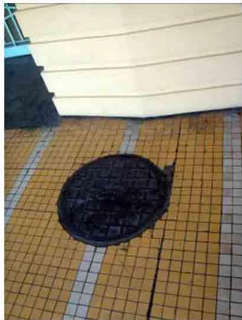
Photo 77. A sewer manhole along the flooring of the sidewalk arcade. Should be cleaned.
