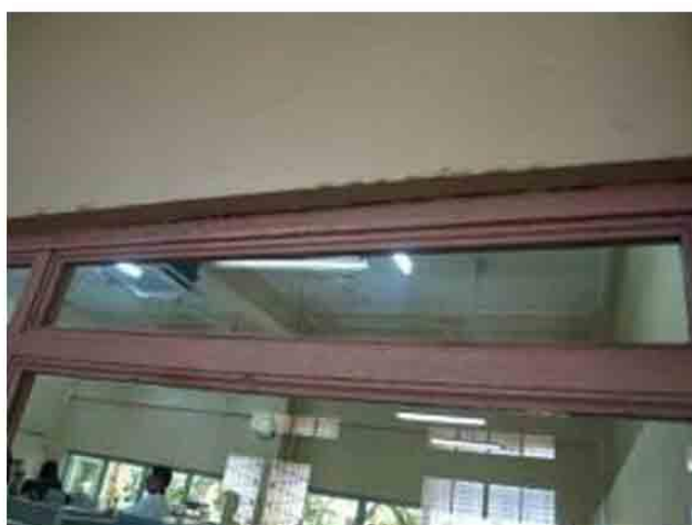
Photo 28. Chipped –off edge of cement plaster finish on top of window
