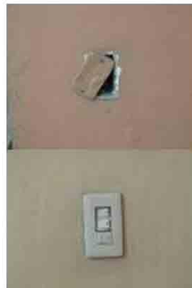
Photo 24. Busted electrical box and electrical switch. Should be repaired or removed if not operational.
