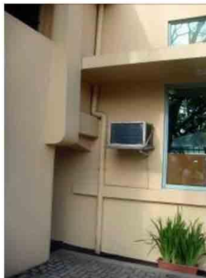
Photo 6. A WACU protrudes at the external envelope of the NRH. New awning glass windows replaced the old ones. Should be covered with grille works to blend with the Art Deco grilles.
