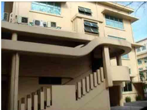
Photo 54. The Art Deco external stairway at the rear right wing of NRH. AC split type condensers are placed at the parapet. Should be provided with Art Deco style grilles to cover.
