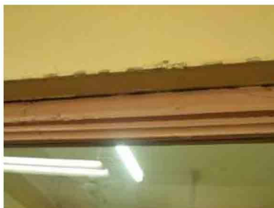
Photo 29. Close-up view of chipped plaster finish. Should be repaired.
