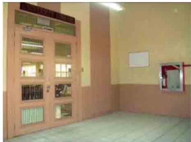
Photo 50. Original Art Deco main wooden door with grille works leading to the University Central Library. Should be preserved.
