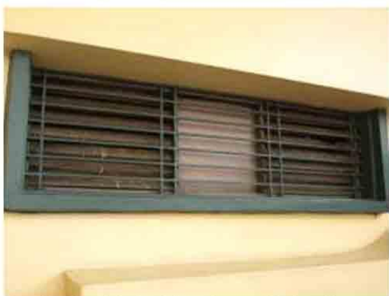
Photo 55. Original jalousie window at the external stairway for ventilation to the kitchen area is blocked off. Should be utilized and cleaned.
