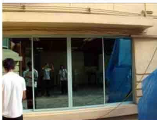
Photo 71. Electrical conduits retrofitted at the exterior right side of NRH. Note newly installed picture window.
