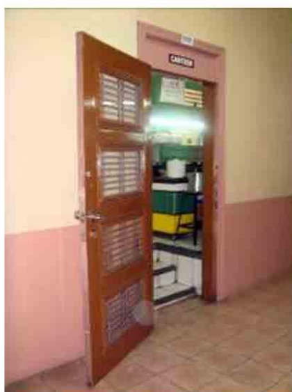
Photo 8. An original swing door with grille works leads to the Canteen at the GF right wing of NRH. Needs refurbishing.
