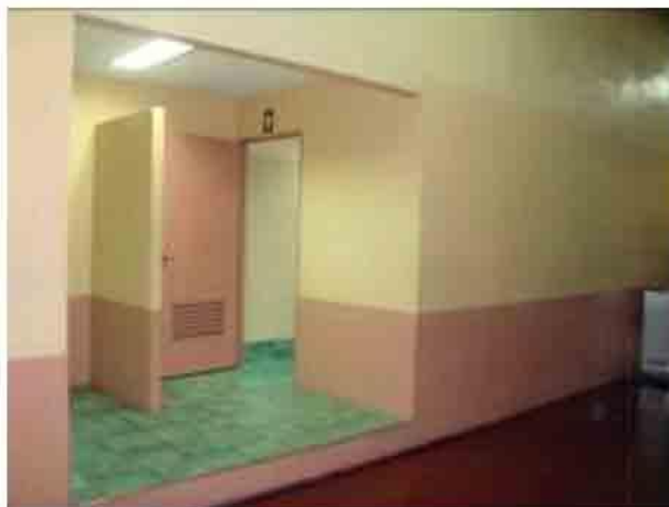
Photo 48. Newly renovated Comfort Rooms (2F, right wing). Note difference of old floor (dark brown) with that of the new (green ceramic tiles). There should be a blend of colors aligned with the finish of the old floor.
