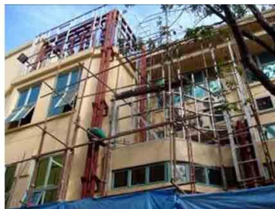
Photo 70. Ongoing construction. Steel framing/cladding is being prepared to cover the heat exchanger pipes being installed.
