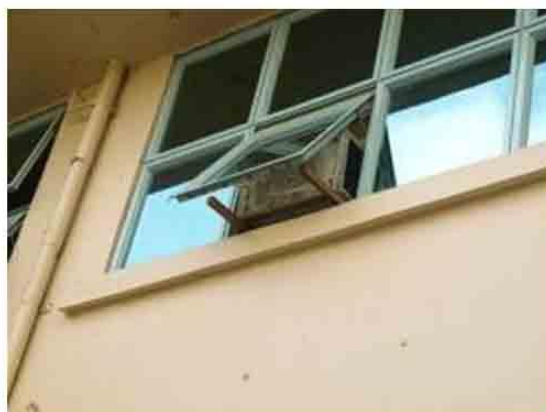
Photo 65. WACU protrudes at the open awning window. Should be relocated.
