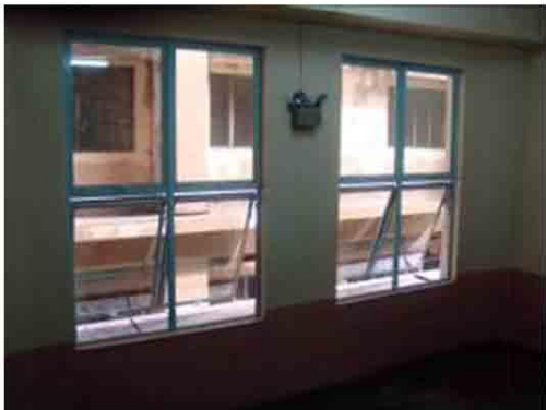
Photo 31. Newly installed awning glass windows at the stairway landing replaced the old ones.
