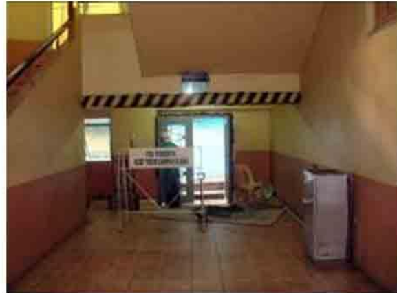
Photo 12. An original Art Deco side door entry being refurbished (Feb. 9'09). An overhead safety buffer (yellow and black stripes) was placed at the edge of the stairway landing because of the low height clearance of floor to stairway landing slab.
