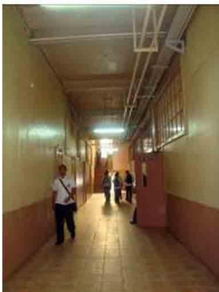
Photo 26. Utility pipelines and ducts align the hallway ceiling. Should be covered discreetly.
