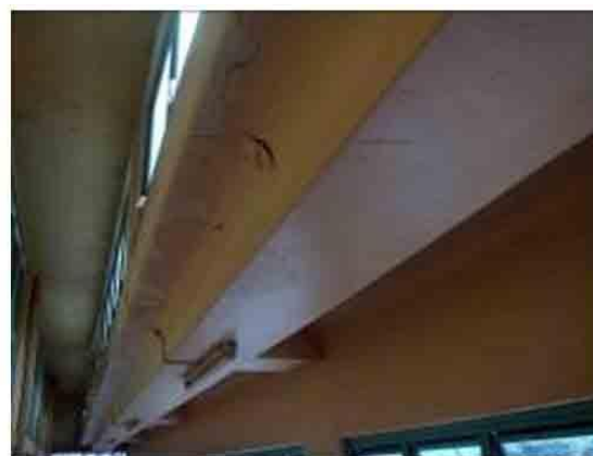
Photo 39. Close-up view of existing cracks and peels. Should be restored.
