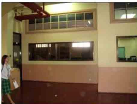
Photo 43. The E-Library extension (an academic classroom before – 1980). Original wooden glass high windows retained and should be preserved.
