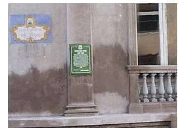
Figure 21: Stain in the Bme. Mitre Façade, 2008
