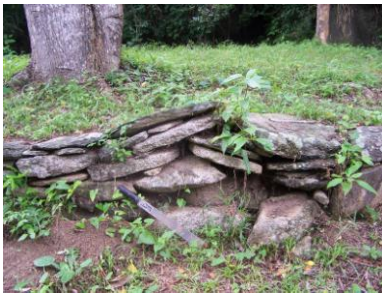
Figure 15. Elements displaced due to the output of roots.
