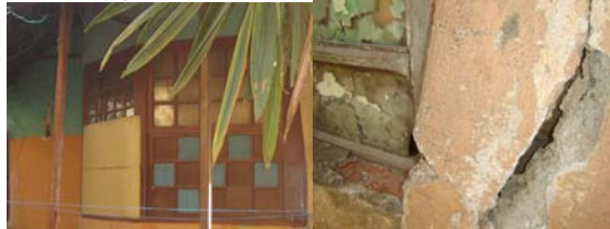
Left: Brocken glasing on windows replaced by wooden and card oards
