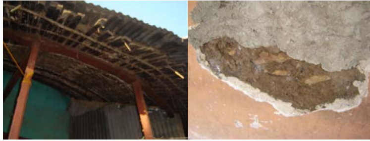
Figure 4: Expected needs of repair: top Left - hand rails on the veranda, top right -fire place bottom left- reed ceiling, bottom right-crack on walls due to the introduction of Cement mortar.
