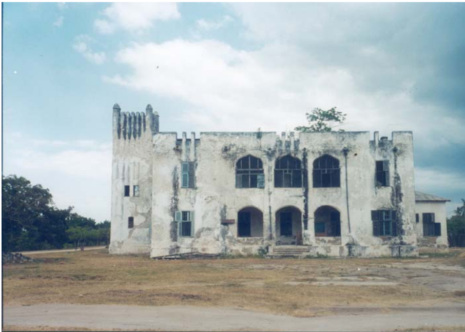
Figure 3: Right Side View of the Old Boma before the collapse of the Balcony
