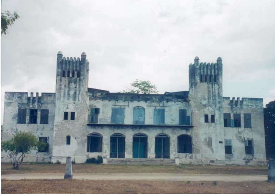
Figure 8: Front View of the Boma after the collapse of the Balcony
