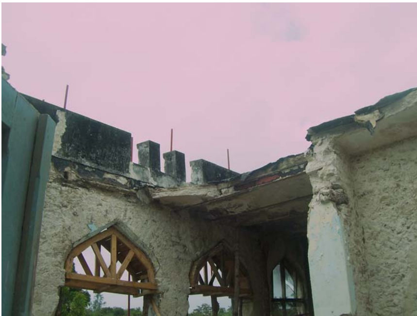
Figure 16: Fraction of Collapsed Flat Roof
