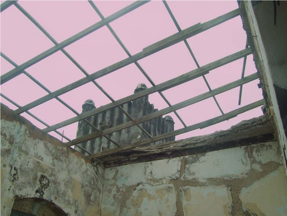
Figure 17: Part of Collapsed Flat Roof to be replaced with Pitched Roof
