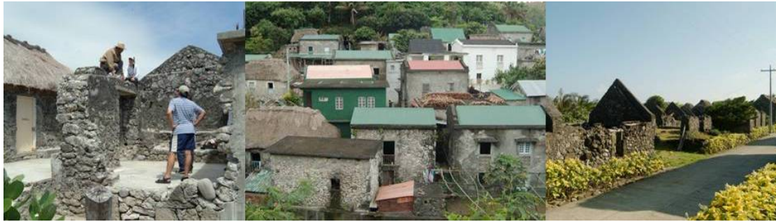
Fig. 25 to 27 - Damage and Changes in the Use of Materials
