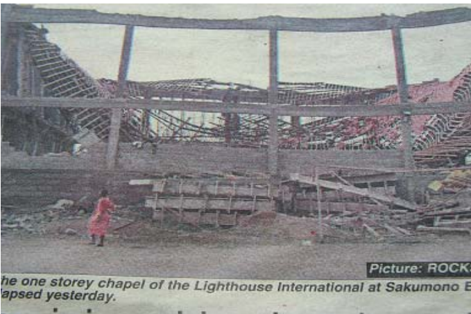
Figure 5. A scanned copy of a news paper publication of a Church which collapsed on a Sunday morning before worshipers came to church.
