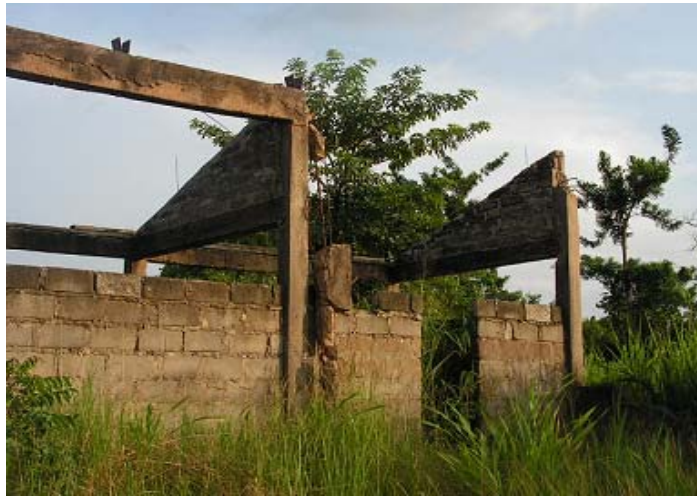
Figure 1. The Remains of a Church building which failed during construction
